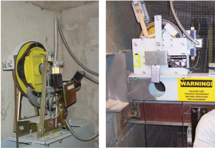
Figure 8: Governors at top of the hoistway; image courtesy of Delaware Elevator
