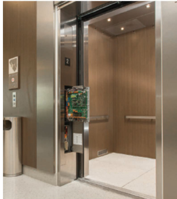
Figure 9: Inspection and test panel; image courtesy of Otis
