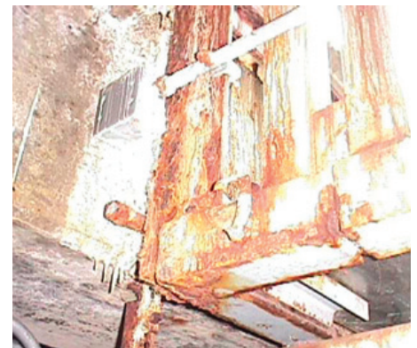
Corrosion on escalator truss and bearing supports due to water
