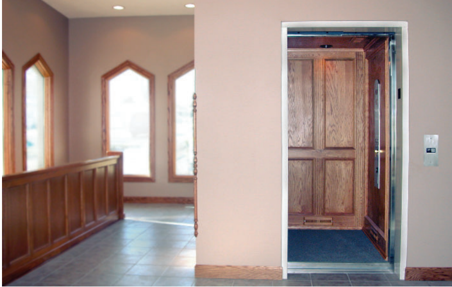
A LU/LA elevator with wood interior
