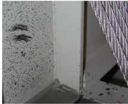
Figure 3: Throw-off (at left) is more than a messy nuisance in the machine room. It can impact proper brake function.
